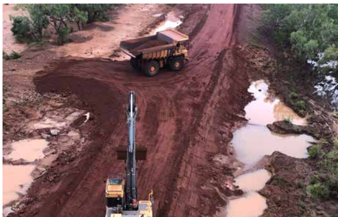
Repairing the Great Northern Highway at Willare as part of the Kimberley Flood Response
