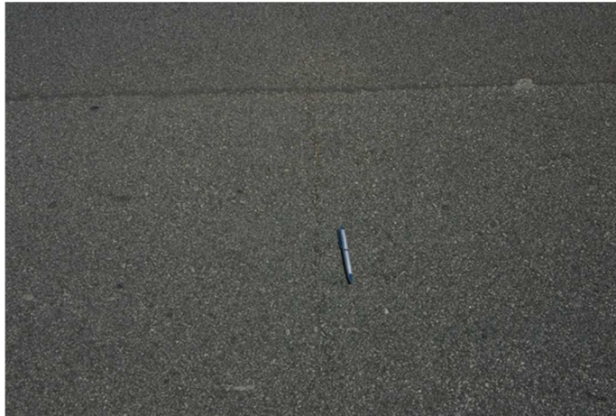
Figure 8: Warton Road – City of Gosnells (January 2012) Transverse crack in asphalt surface on CRC base
