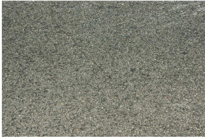
Figure 6: Welshpool Road –CRC section showing transverse crack (January 2015)
