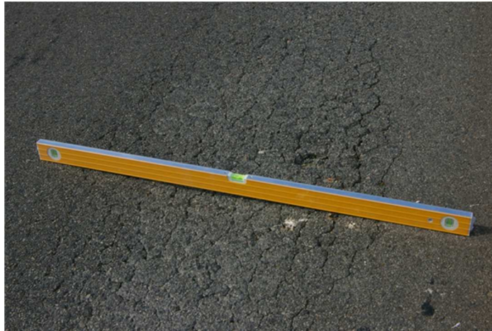
Figure 3: Gilmore Ave showing one of many fatigue failed sections in the CRB control section (January 2011)
