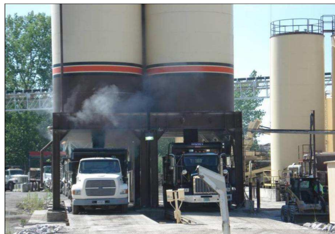
Figure 20 Fuming of HMA on left and no fuming of WMA on right
