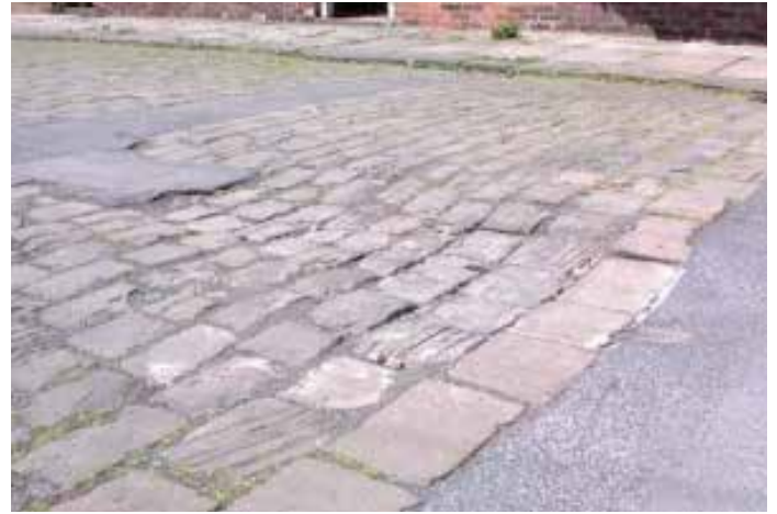
Subsidence of pavers
