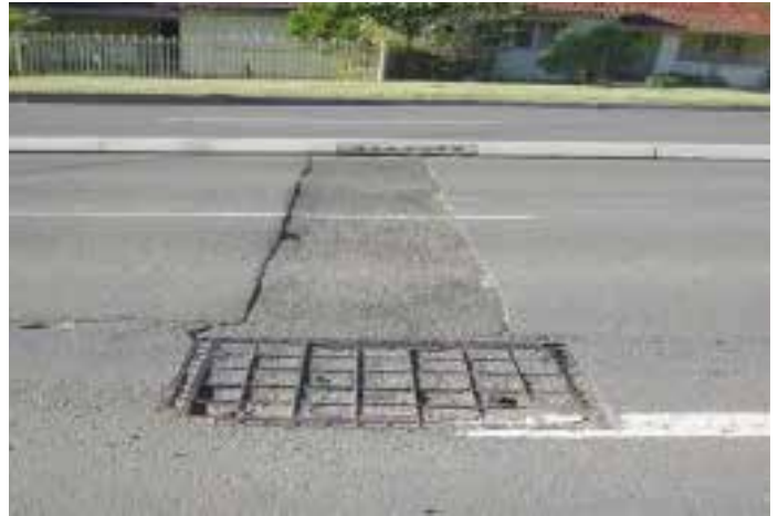
Poor trench repair
