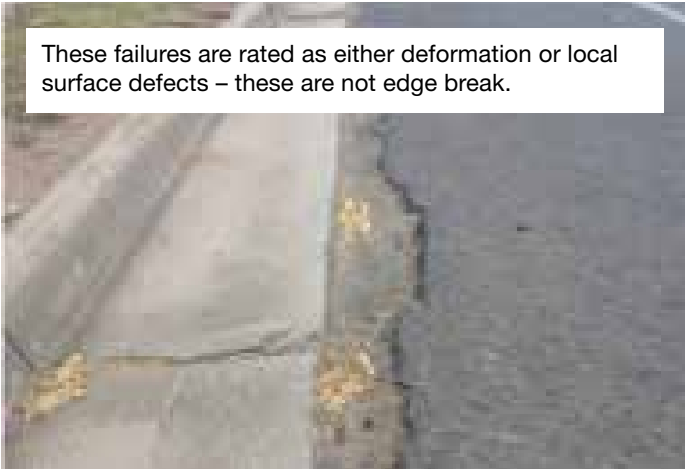
Failure at edge of seal and channel
