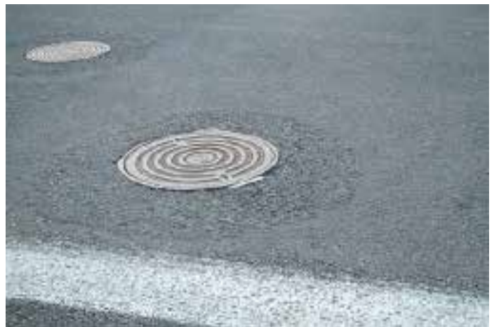
Poor patch repair
