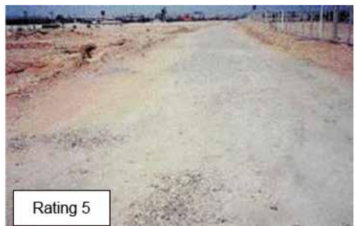
Evidence of protrusion
