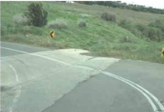
Poor water channel construction
