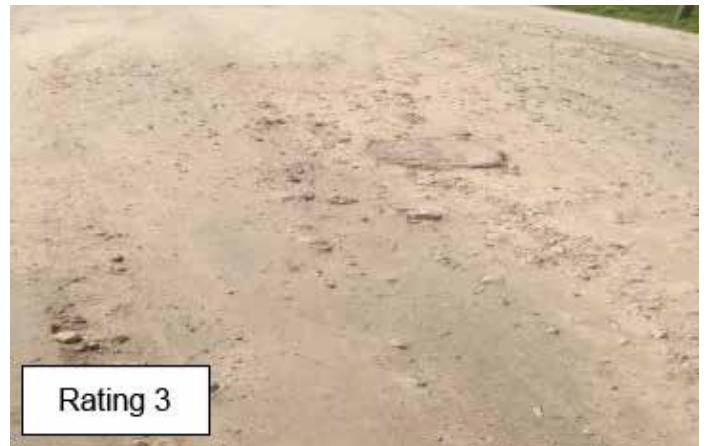
Evidence of scattered protrusion
