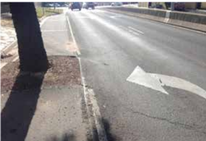
Tree root causing up-heave
